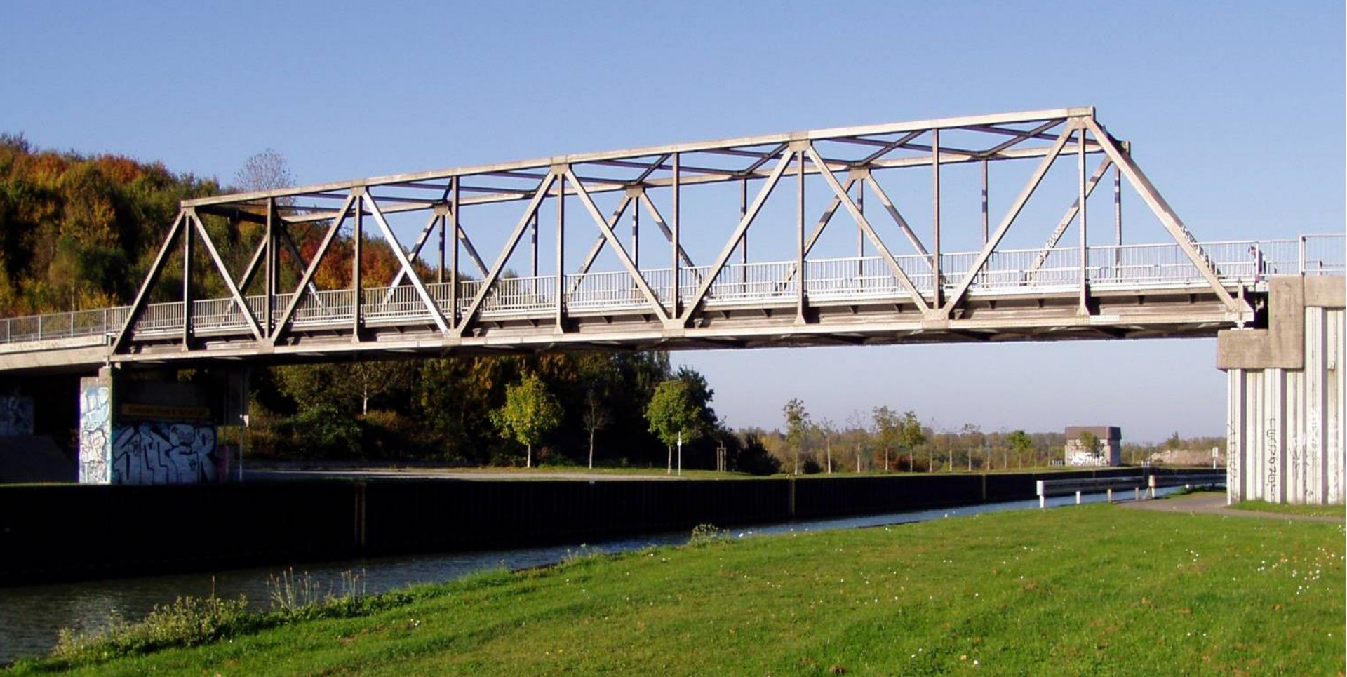
Schwansbell Bridge, Lünen - built in 1956 (Photo: 2005) Profiles, sheets, rivets: AlMgSi1 - mill finished
