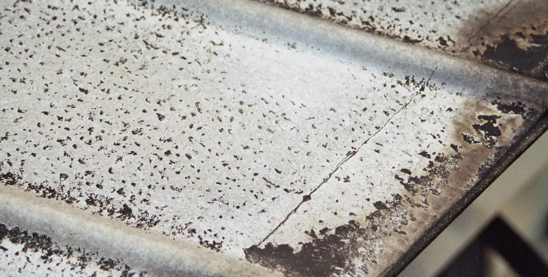
Dortmund Westfalenhalle Condition of the roof in 2007
