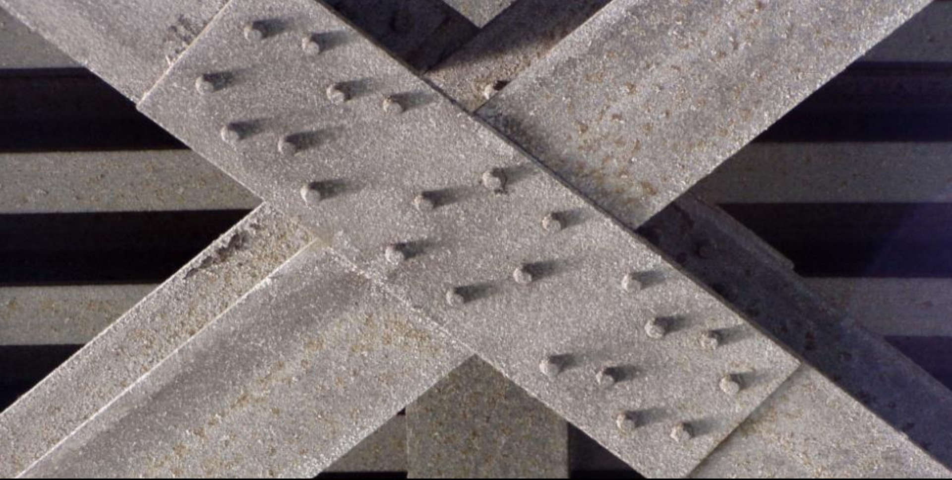
Schwansbell Bridge, Lünen - built in 1956 (Photo: 2005) Profiles, sheets, rivets: AlMgSi1 - mill finished
