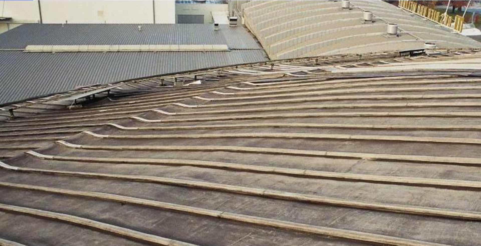
Dortmund Westfalenhalle Condition of the roof in 2007
