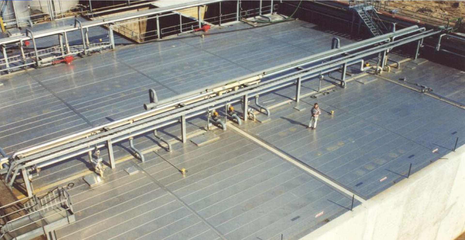
Basin cover in a sewage treatment plant
