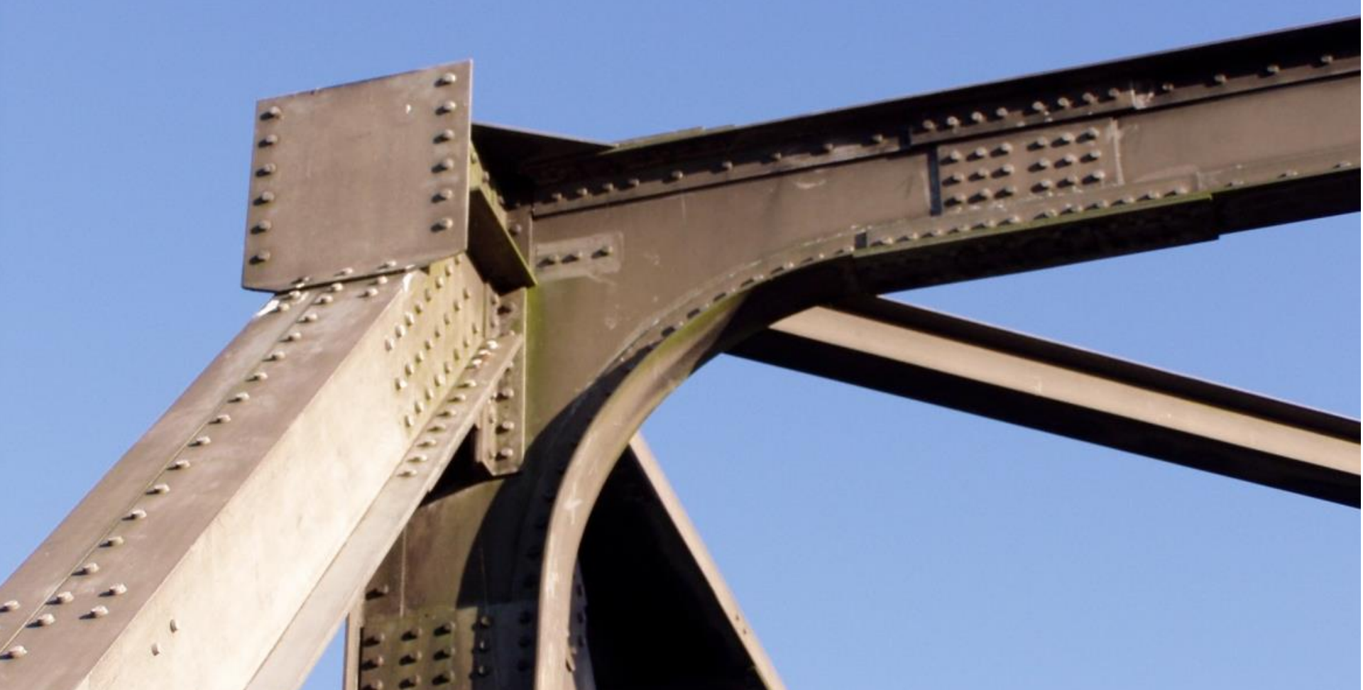
Schwansbell Bridge, Lünen - built in 1956 (Photo: 2005) Profiles, sheets, rivets: AlMgSi1 - mill finished
